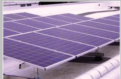
The Center's photovoltaic cells reduce energy costs by $22,000 annually.
